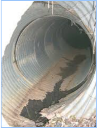
Storm pipe offset
