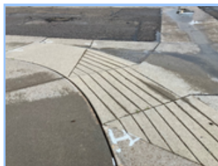
Sidewalk Ramp Tripping Hazard
