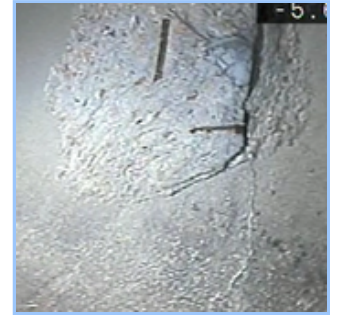
Storm pipe with hole 3
