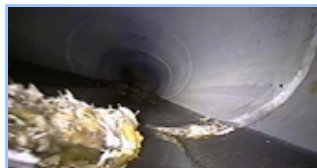
storm pipe with debris
