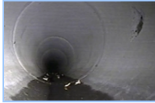
Storm pipe with hole
