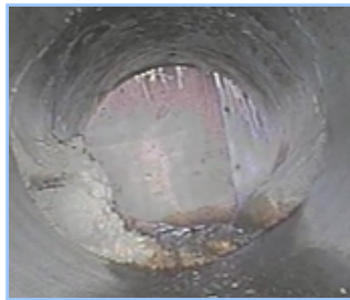
storm pipe with excess grout
