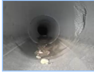
Storm pipe with hole 2
