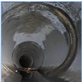
storm pipe with joint separation 3
