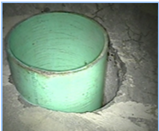
Storm pipe with protruding tap
