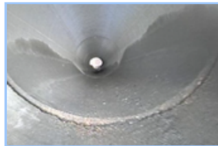
storm pipe with joint separation
