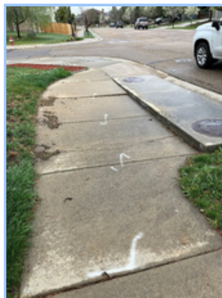
Unlevel with Storm Drain
