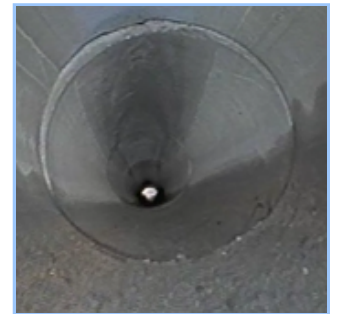
storm pipe with joint separation 2
