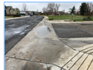
Cracked Drain Pan
