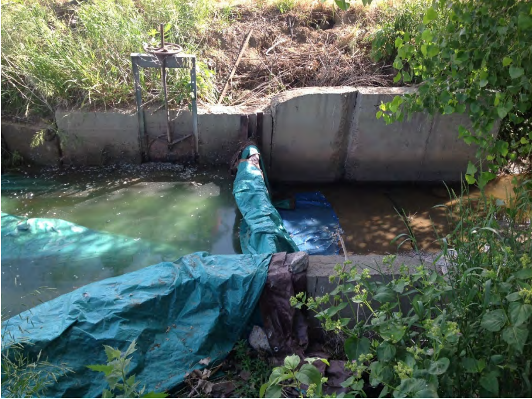
Modern headgate in use at 5WL2248.14, facing northeast.
