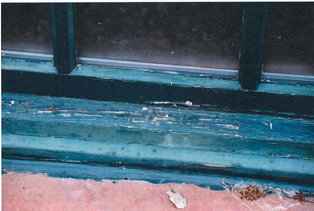
Lincoln School: Detail of Deteriorating Window Sill
