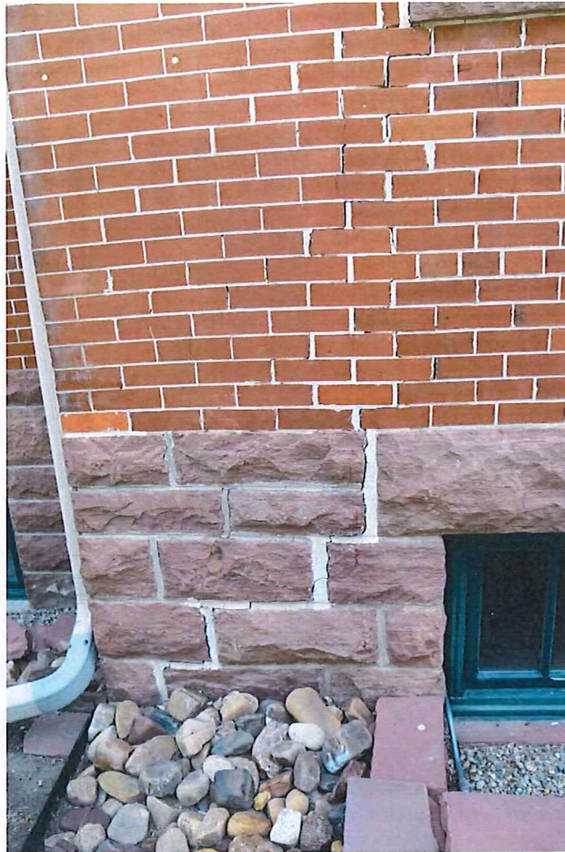
Lincoln School: Detail of Corner Settlement and Repair
