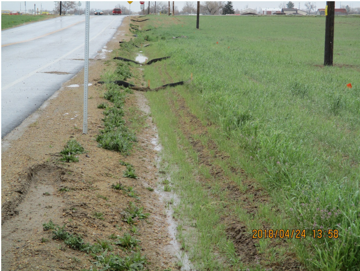
Photo 4: Photo of the roadside ditch along the northern boundary of the Survey area along Weld County Road 6.
