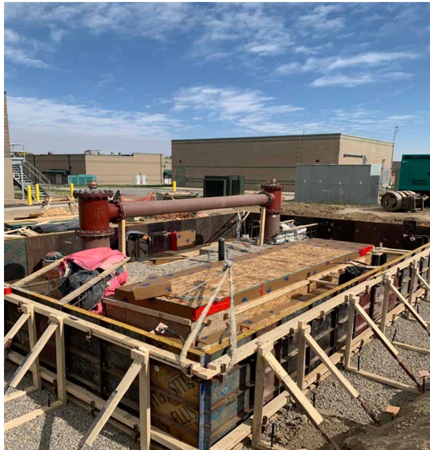
Hydroturbine foundation and piping
