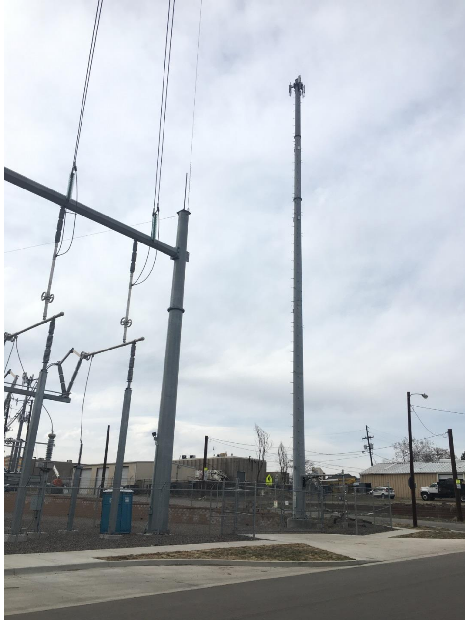
Picture of Argo FAN Tower (looking NW)
