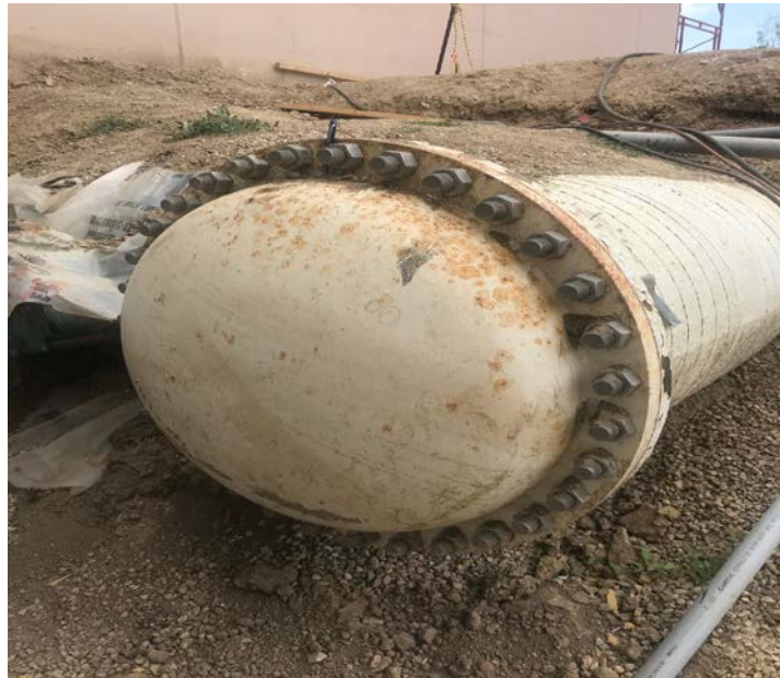
36 inch pipe from raw water to pre-treatment
