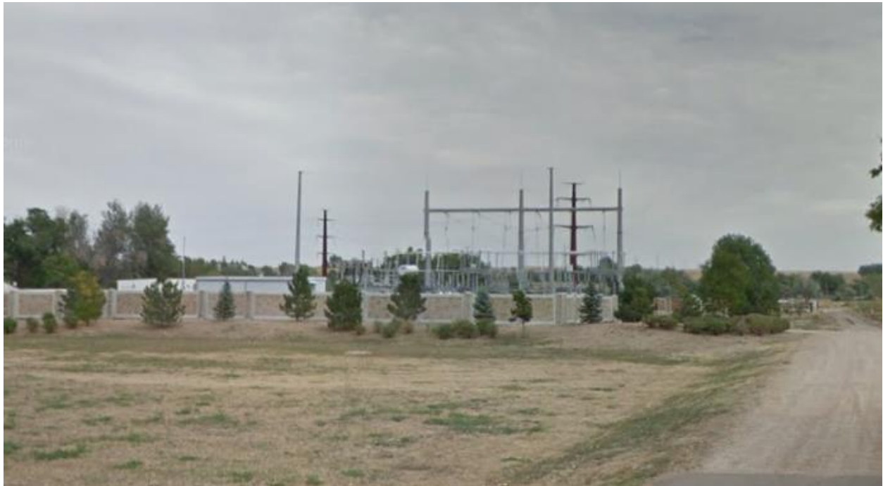
Figure 2. View of Isabelle Substation, Looking to the East.
